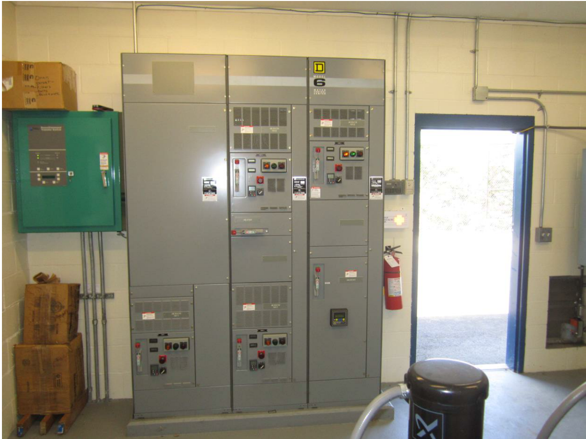
Panorama Booster Pump Station
